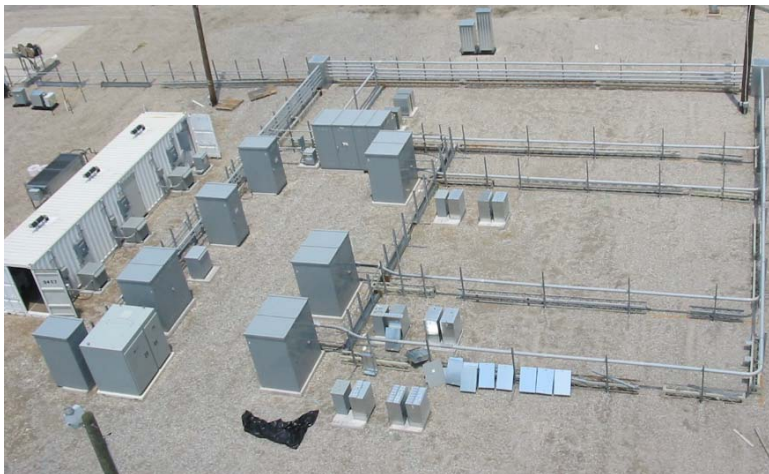
CERTS Microgrid Test Bed at American Electric Power
