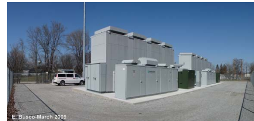
Sodium Sulfur Battery 2 MW
